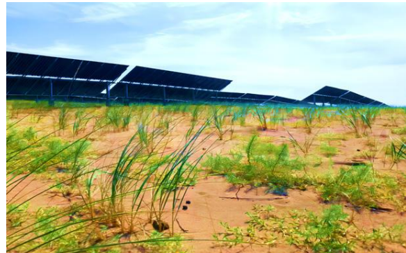
Solar Panels Installed in Badain Jaran Desert
